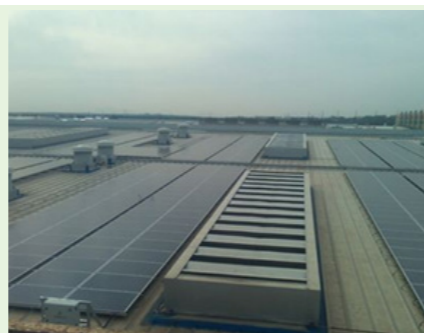
Dongjiakou plant's photovoltaic facilities
